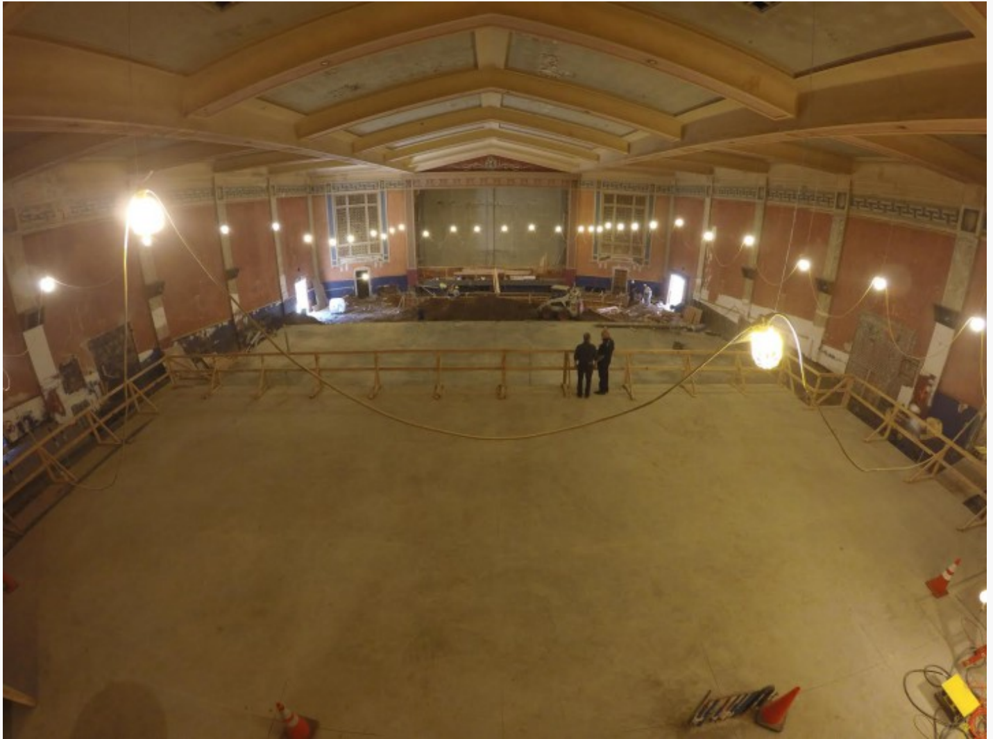
The push to renovate the UC Theater on University Avenue got a huge boost after a major philanthropist made a $1.3 million matching grant. Photo: UC Theatre
